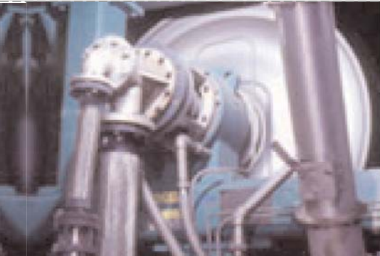
The dryer section of a high-speed papermaking machine.
